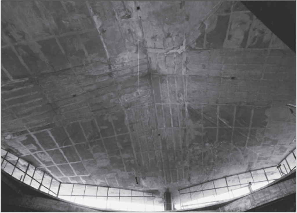
This mid-1961 interior view shows the roof before final plastering and painting, looking up from the library's rotunda.
