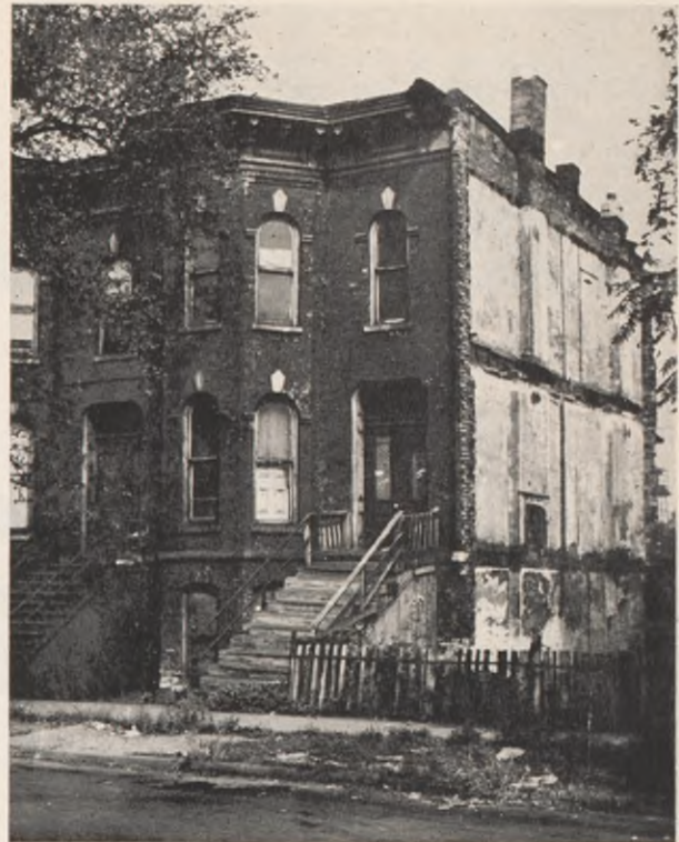
A typical depreciated building
