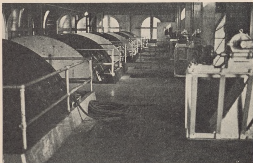
FIG. 3. Inside of Screening Plant at Hyperion.
