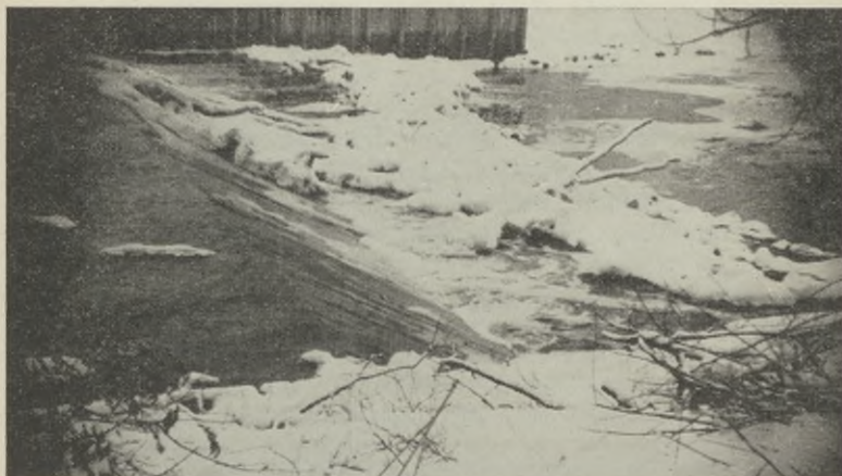
Riverside Park Dam at Station 6 in Grand Forks. A typical Low Overflow Dam.
