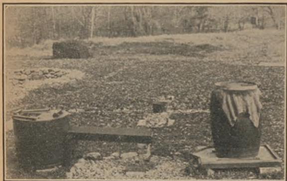
FIGURE 30.—Soakage pit and grease traps. Left, cold water grease trap; right, ash barrel grease trap.
