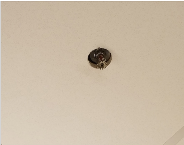
Fire sprinkler head missing metal plate
