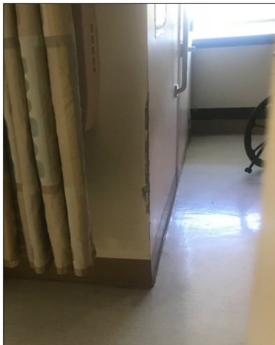
Wall corner with damaged plaster and paint
