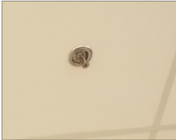
Fire sprinkler head with proper configuration
